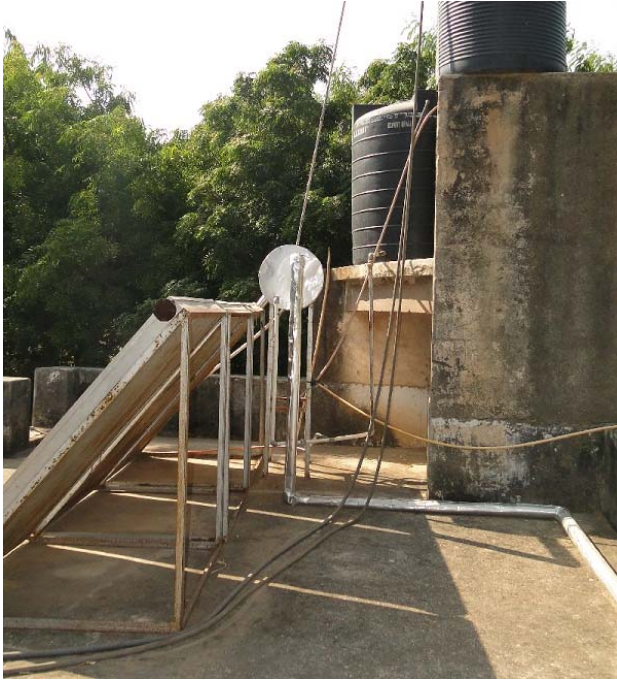
Fig. 10 : Solar Thermal System installed at Tilonia*
